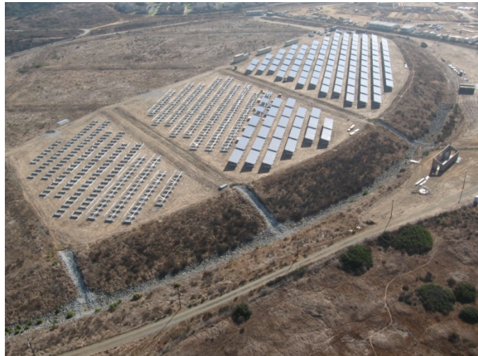
Figure 1. PV system incorporated into IR Site 7 landfill cap, Marine Corp Base Camp Pendleton
